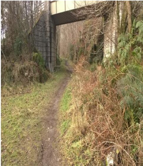
The Lochearn Railway Path is a good example of an upgrade to an existing off road facility to improve usability for cycling and wheeling. The project was funded by NatureScot and Sustrans.
